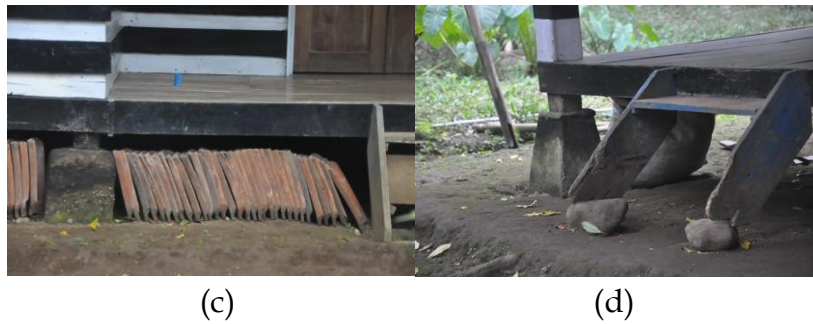
Figure 10. Foundation Construction. (a) form of Pasagi foundation; (b) the shape of the Lisung foundation; (c) the function under the house is to become a roof storage area; (d) steps to access the house (Author Documentation)
