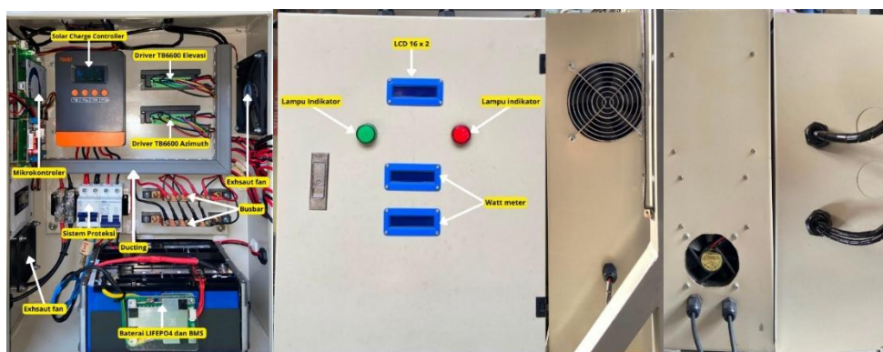
Figure 6. Solar Tracking Control Box Panel Source : Personal Documents
